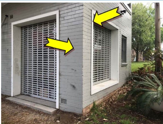
Photo 5. Exterior, throughout, walls and frames – suspected lead-containing grey and white upper coloured paint systems.
