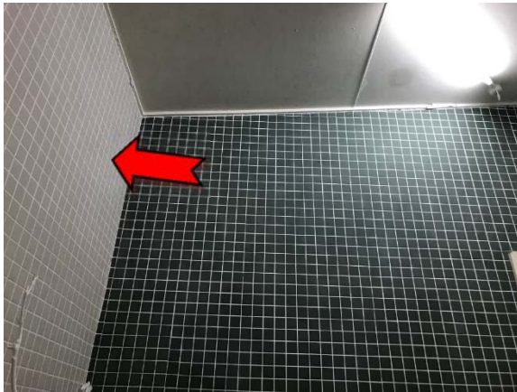
Photo 3. Interior, bathroom, walls – suspected asbestos-containing fibre cement sheeting
