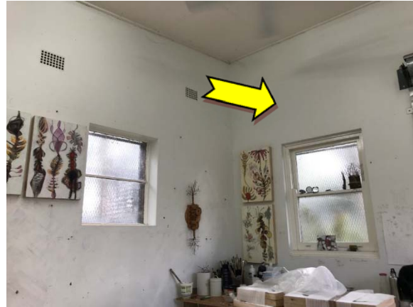
Photo 8. Interior, throughout, walls – suspected lead-containing grey upper paint systems.
