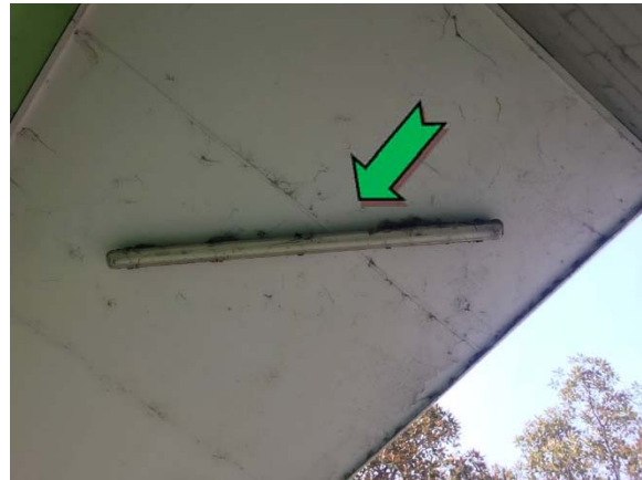
Photo 4. Exterior, throughout, single tubed fluorescent light fitting – suspected non PCB-containing capacitor.
