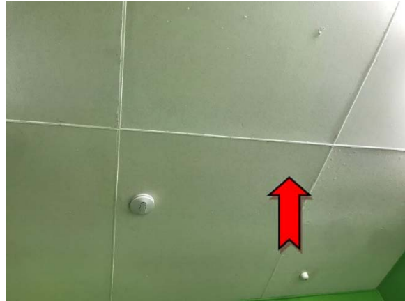
Photo 2. Interior, throughout, ceiling – asbestos-containing fibre cement sheeting.
