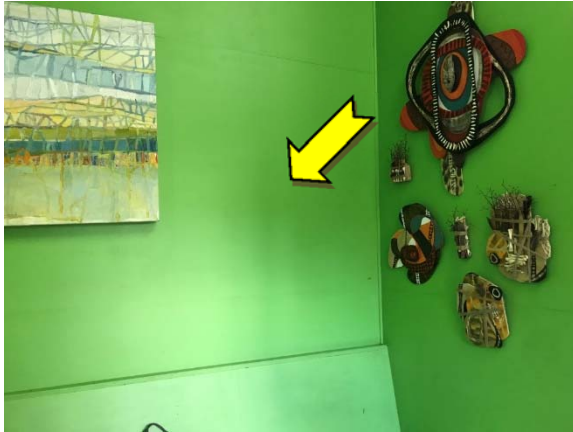
Photo 7. Interior, throughout, walls – suspected lead-containing light green upper paint systems.
