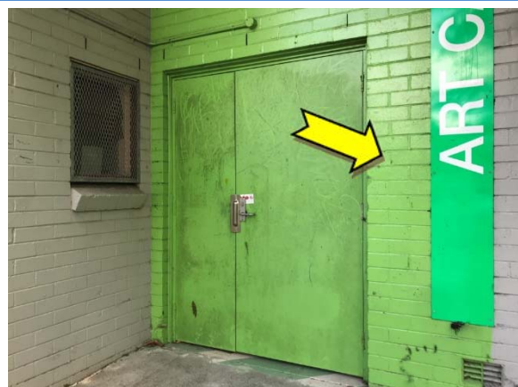
Photo 6. Exterior, throughout, feature wall – suspected lead-containing light green upper paint systems.
